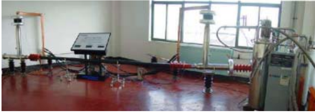
Figure 4. The photo picture of the 4-meter superconductor cable system.
