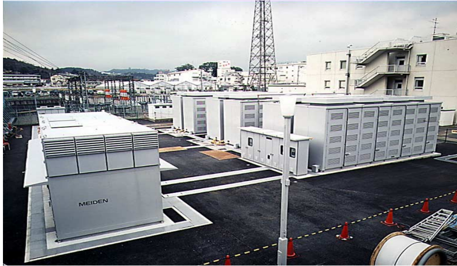
Figure 8-8 6MW, 48MWh NAS System at TEPCO's Ohito Substation (Courtesy TEPCO)
