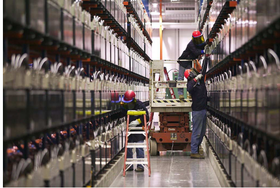
Figure 7-5 GVEA BESS NiCd Battery (Courtesy GVEA)
