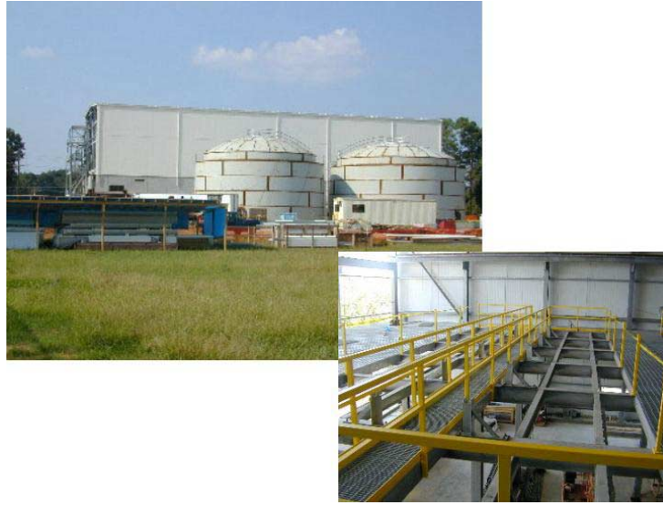
Figure 11-8 Exterior and Interior Views of Progress With Construction of Regenesys Energy Storage Plant at Columbus Air Force Base Site
