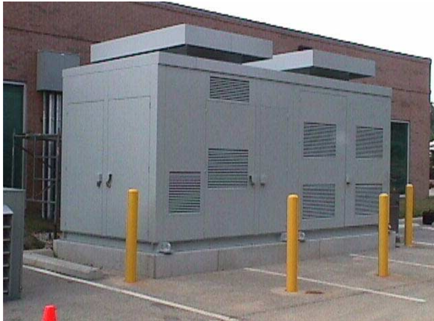
Figure 8-10 AEP's 500 kW ac (PQ) / 720 kWh ac (PS) NAS Unit (Courtesy AEP)
