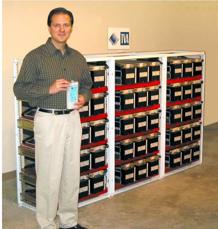
Figure 14-18 Demonstration 2 kV, 1 MW dc Electrochemical Capacitor String for Mini-FACTS Controller
