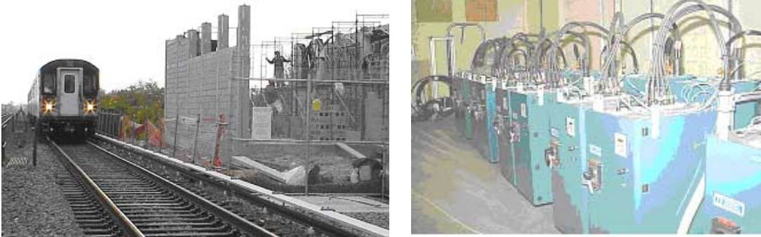
Figure 13-14 Flywheel Installation at NYCT Bay Equalizer Location, 10 100-kW Units in New Building
