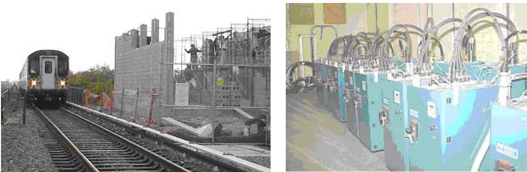
Figure 17 Flywheel Installation At NYCT Bay Equalizer Location, 10 1-MW Units In New Building
