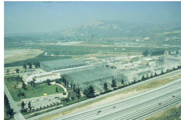
Celilo I/C Station “A Mountain of Silicon”
