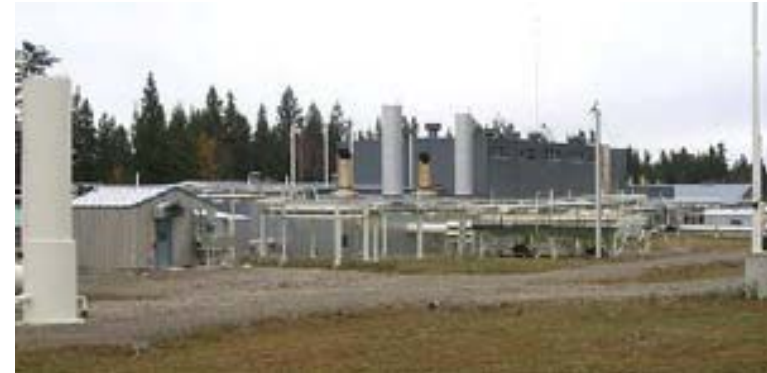
Pumping station for a natural gas pipeline
