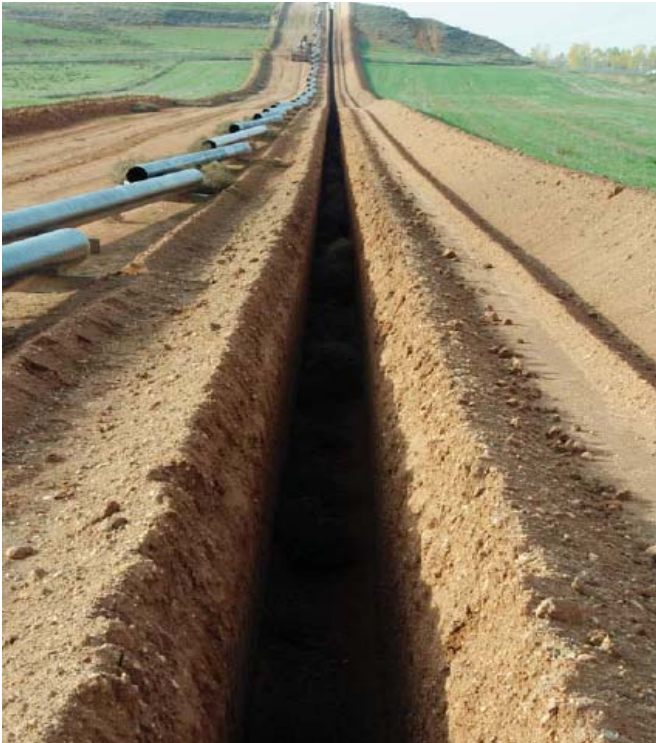
Natural Gas Transmission Pipeline and Pumping Station
