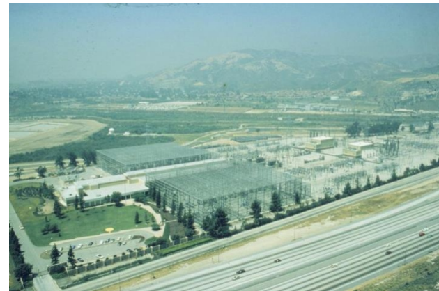
Celilo I/C Station “A Mountain of Silicon”
