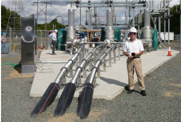
138 KV AC, 574 MW HTS(1G) based (Long Island Power Authority, Nexans)
