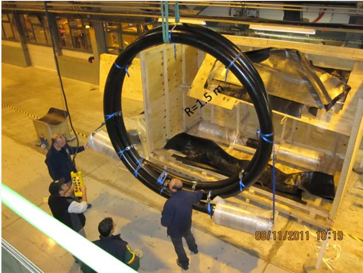
20-m Long Nexans Transfer Line
