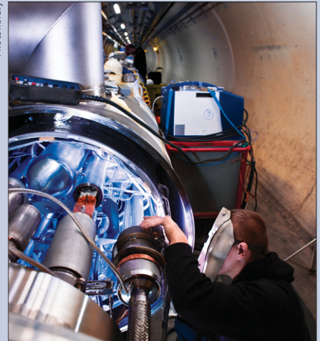
Interconnected A welder works on the junction between two of the LHC’s superconducting magnet systems, in the LHC tunnel.
